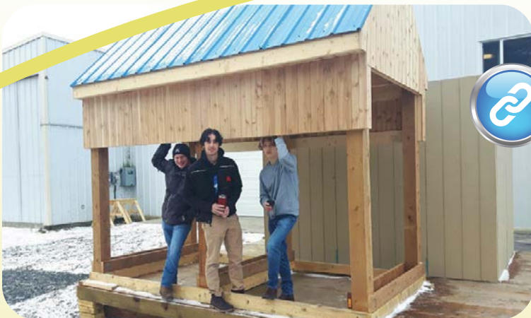
A community partnership will give barn swallows a new place to call home thanks to the St. Thomas Aquinas Grade 12 Construction class. The collaboration between the high school and Ontario Power Generation will give barn swallows near OPG’s Whitedog Falls Generating Station a place to build their nests.
